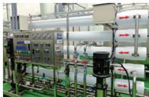
RO membrane system
